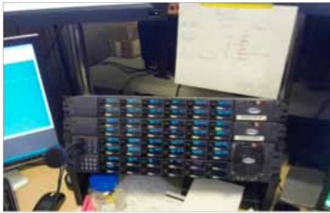
Figure 4: The Comms Control position showing V-Series panels with expansion panels.
